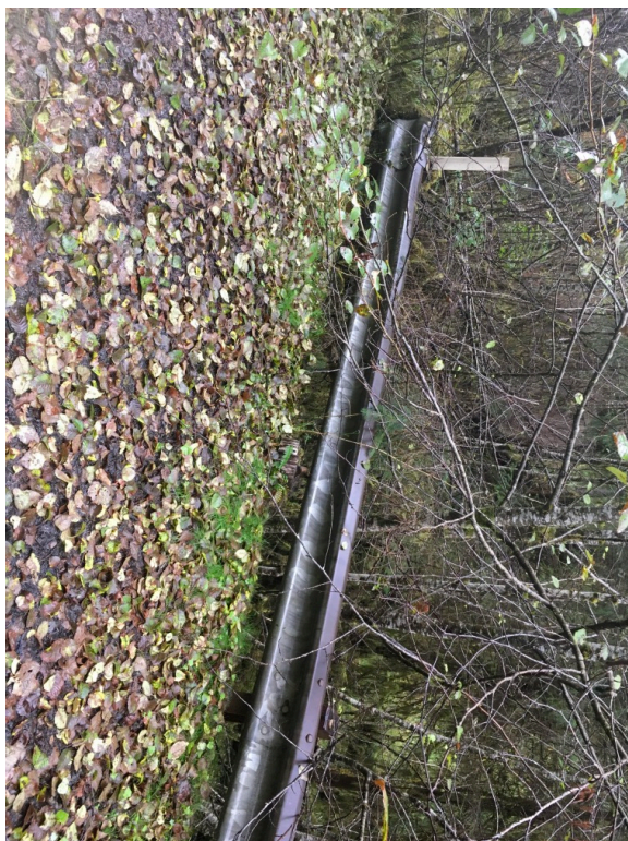
Guard Rail missing riser post
